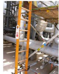
Figure 6: Standard Wooden Ladder used in the plant for temporary access
